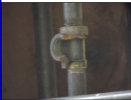
Broken sprinkler pipe in Henderson Building
