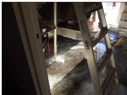
Third floor office where leak occurred
