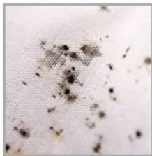
Black or brown stains, usually in crevices
